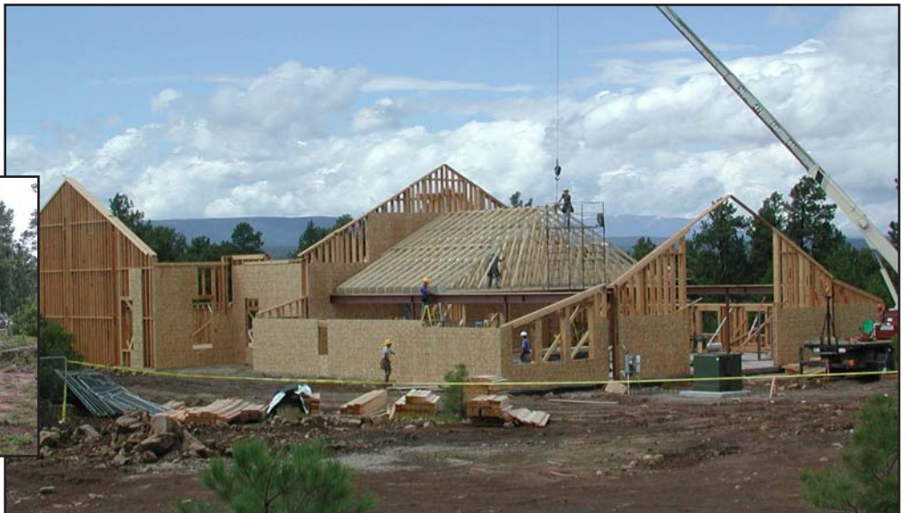
This picture shows that 10 trusses were erected by noon. As of 4:30 p.m., September 10, all the trusses are now in place and ready for the roof to be installed.
