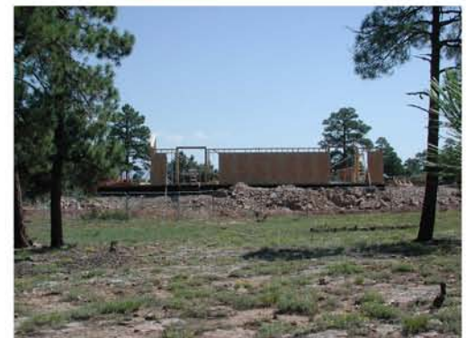
May through August JPPII: land clearing to utilities installation and now to wall framing.
